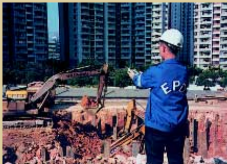
Task force enforcement operation against construction activities in December 1999 caught 78 non-compliance cases
