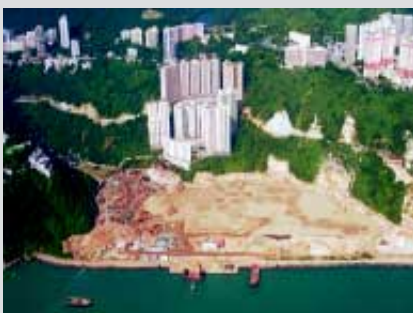
The statutory EIA process allowed due environmental considerations in the planning and design of Cyber Port development
