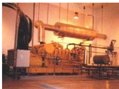
Landfill gas is used to generate electricity
