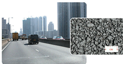
A close look of the low-noise road surface showing the open-texture finish
