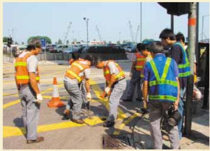
EPD and Drainage Services Department staff jointly investigate a sewer odour problem in Kennedy Town.
