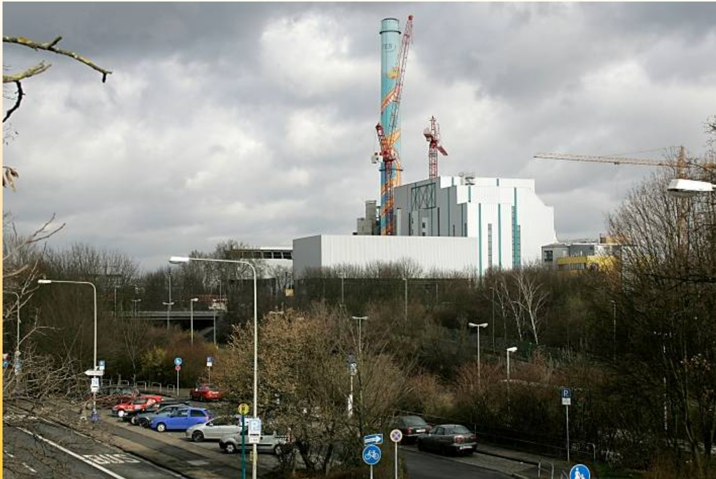
New Boiler House
