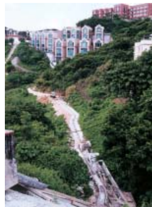
銀線灣區的渠務工程 Construction of sewerage system for the Silverstrand area
