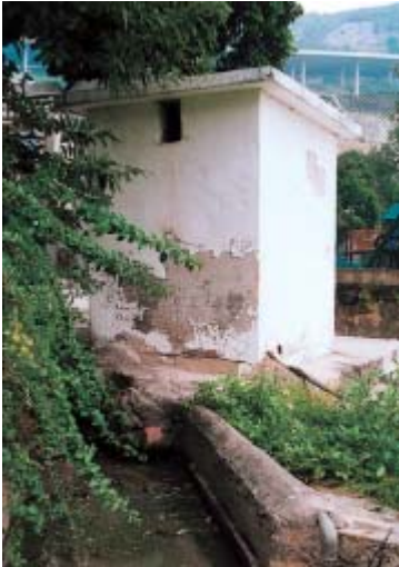
汀九泳灘的次氯酸鈉劑量調控系統 The hypochlorite dosing system at Ting Kau Beach
