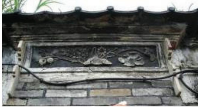
Façade Wall Frieze Decorative Feature of the First Bay from the Easternmost End
