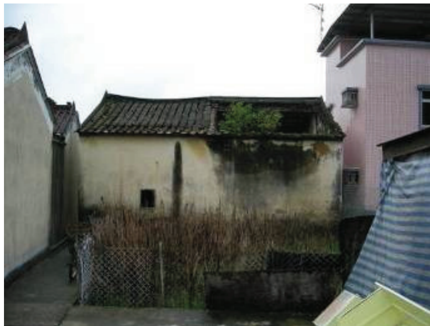
Back view (collapsed roof)
