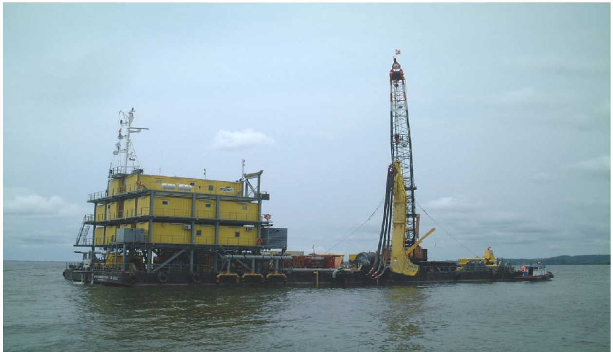
Cable laying barge with injector tool 裝有注射工具的光纜鋪設躉船
