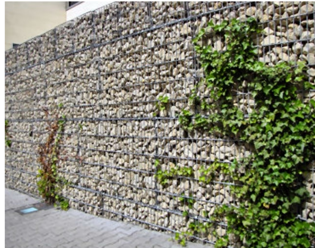
PREVIOUS EXAMPLES OF DEFLECTOR WALL WITH GABION BLOCK FOR NATURAL TERRAIN HAZARDS MITIGATION WORKS 用於防治山泥傾瀉工程導流牆及石籠例子
