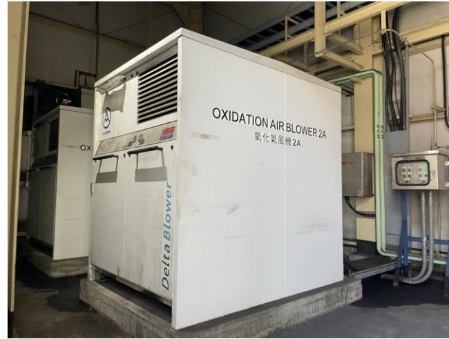
Photo 68: The oxidation air blower units of the FGD plant with oil stains observed 照片 68：煙氣脫硫裝置的氧化吹風機 (觀察到有油漬)
