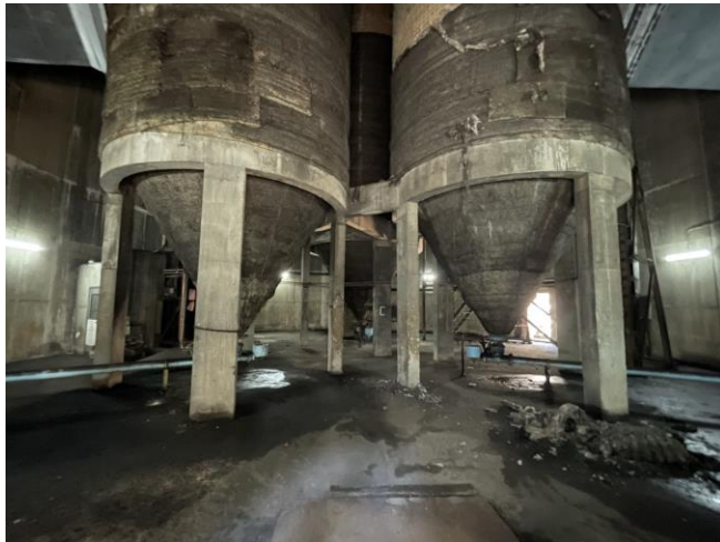
Photo 70: Inside view of the chimney with mixture of dirt and stagnant water observed 照片 70：煙囪內部視圖 (觀察到有污垢和積水的混合物)
