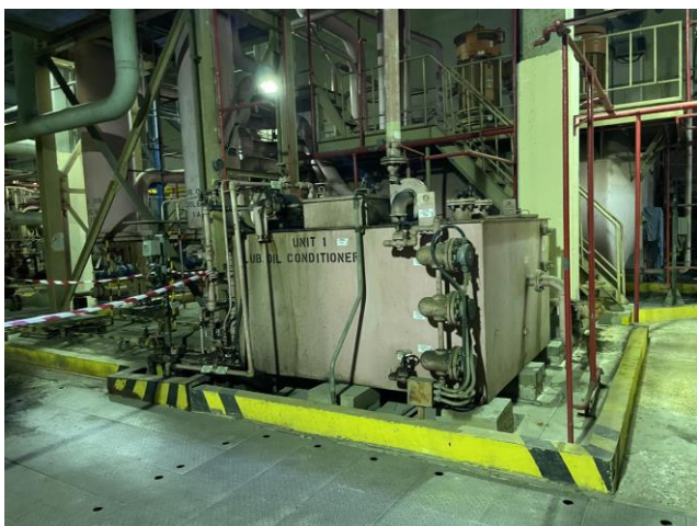
Photo 28: Lubrication oil conditioner and coolers at L1 照片 28 : L1號機組的潤滑油調節器及冷卻器
