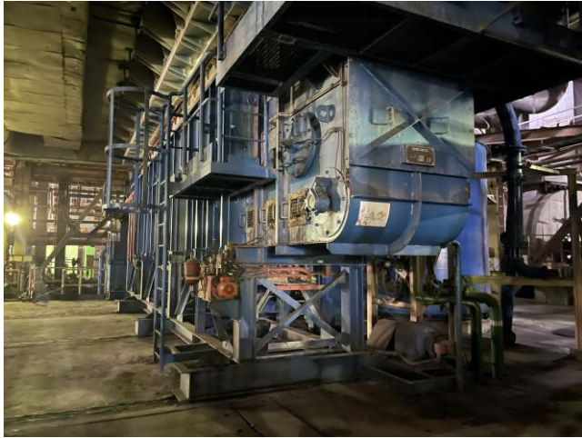
Photo 7: Boiler area and submerged scraper conveyor 照片7：鍋爐區及水下刮板輸送帶
