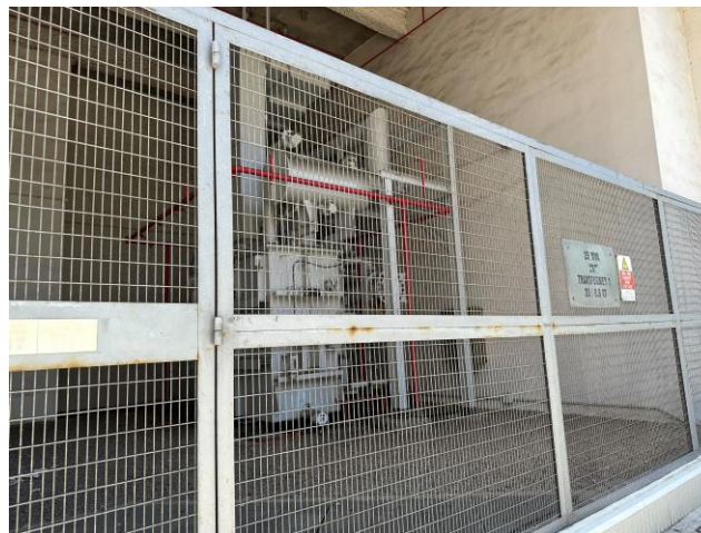
Photo 47: Transformer along the Main Station Building for L1 to L3 照片 47：沿L1至L3號機組的主廠房大樓的變壓器
