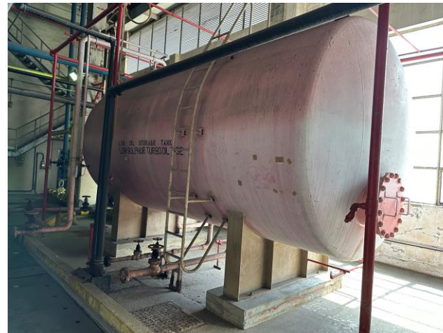
Photo 23: Lubrication oil storage tank 照片 23 : 潤滑油貯存缸
