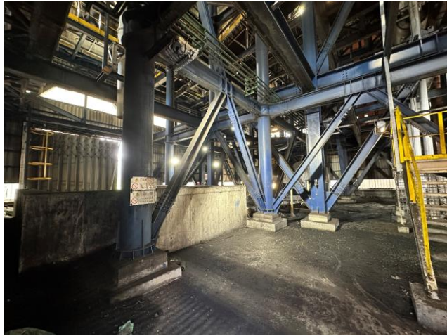
Photo 91: Inside of Junction Tower T16, coal pieces and mixture of coal residuals on ground 照片 91 : T16號接駁塔內部, 地上的煤塊和煤渣的混合物)
