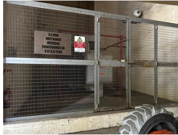
Photo 59: Transformer along the Main Station Building 照片 59 : 沿L1至L3號機組的主廠房大樓的變壓器
