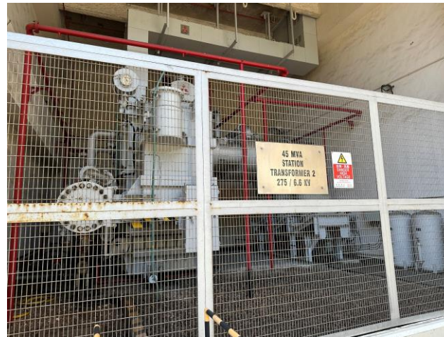
Photo 53: Transformer along the Main Station Building 照片 53 : 沿L1至L3號機組的主廠房大樓的變壓器
