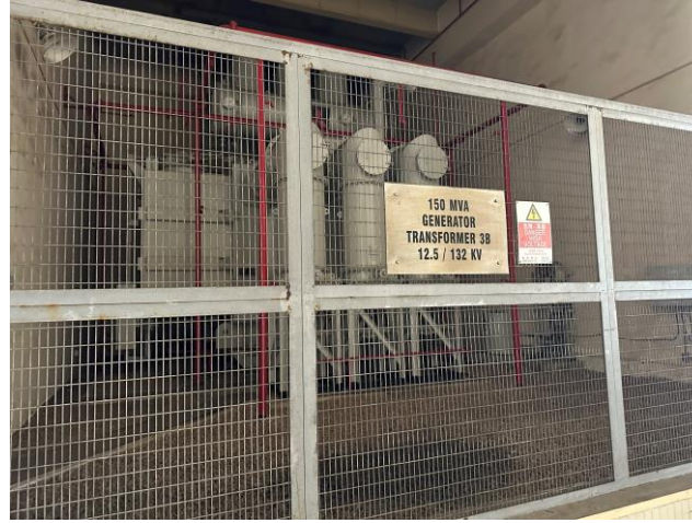
Photo 56: Transformer along the Main Station Building 照片 56 : 沿L1至L3號機組的主廠房大樓的變壓器
