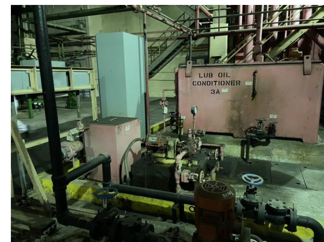
Photo 30: Lubrication oil conditioner, oil pumps and sump pit at L3 with oil stains observed 照片 30 : L3號機組的潤滑油調節器, 油泵及集水坑(觀察到有油漬)
