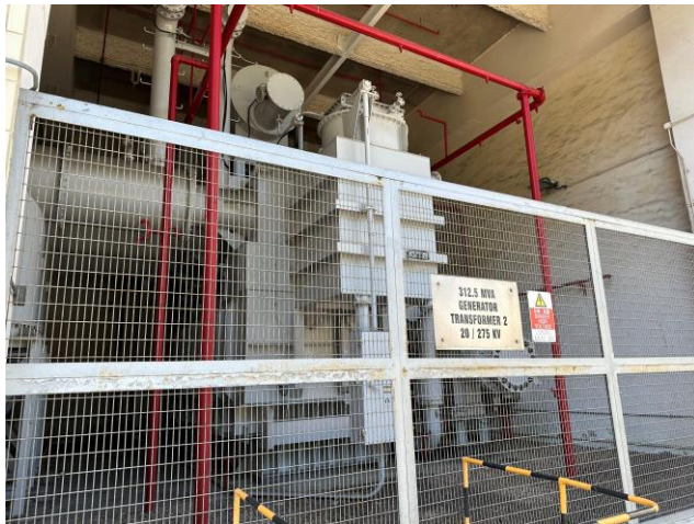
Photo 52: Transformer along the Main Station Building 照片 52 : 沿L1至L3號機組的主廠房大樓的變壓器
