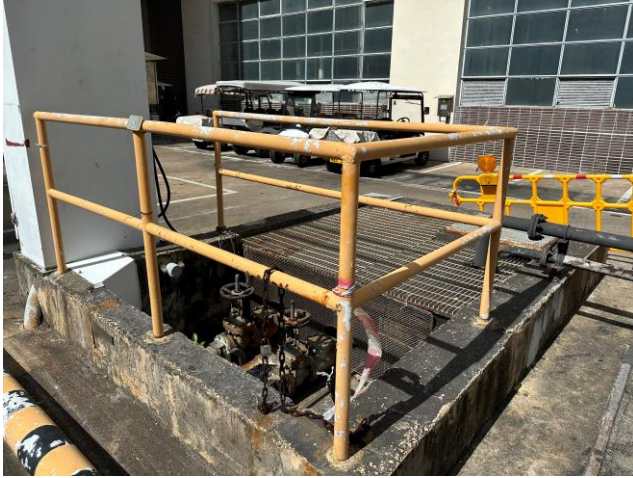
Photo 61: The oily drain sump outside the Main Station Building for L1 to L3 照片 61：L1至L3號機組的主廠房大樓外的油脂渠集水坑
