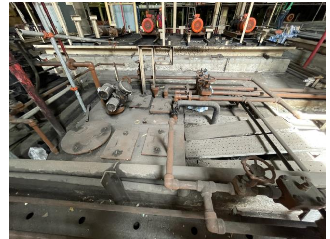
Photo 12: A fuel oil drain tank 照片12：燃油排放缸
