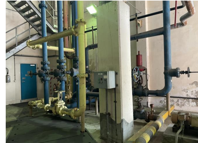
Photo 24: Oil transfer pump 照片 24 : 輸油泵
