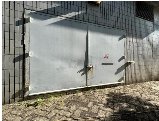
Photo 89: Transformer room in the GT57 & Coal Jetty Electrical Equipment Building 照片 89 : GT57及煤船碼頭電氣設備大樓內的變電房
