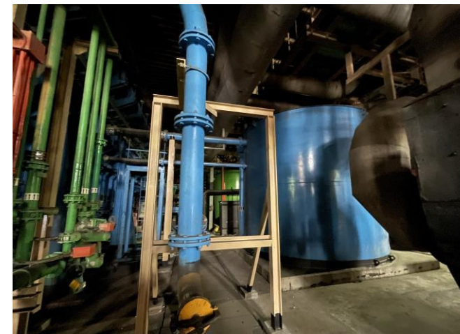
Photo 42: Water tank and overflow water tank 照片 42：水缸及溢流水缸
