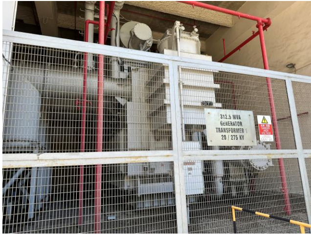
Photo 49: Transformer along the Main Station Building 照片 49 : 沿L1至L3號機組的主廠房大樓的變壓器
