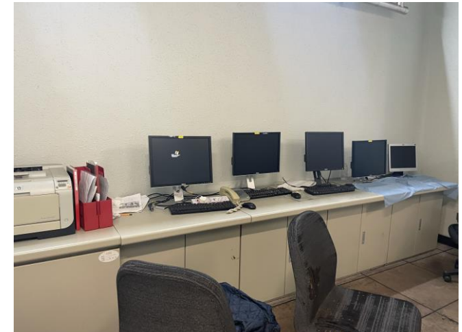
Photo 78: Control equipment room in Unit 2 FGD Electrical and Control Equipment Building 照片 78 : 二號煙氣脫硫裝置電氣及控制設備機樓的控制設備室
