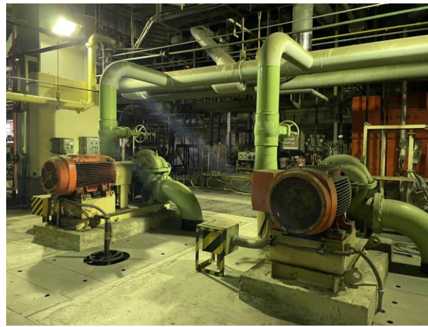
Photo 44: Bearing cooling water pump 照片 44：軸承冷卻水泵
