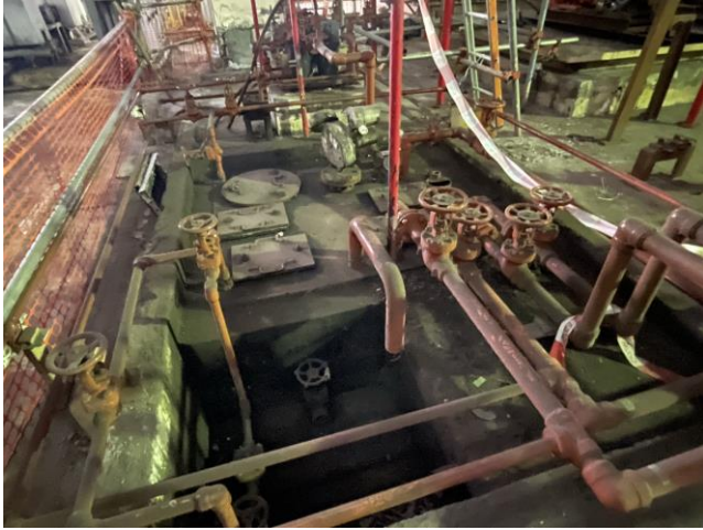
Photo 13: A fuel oil drain tank 照片 13 : 燃油排放缸
