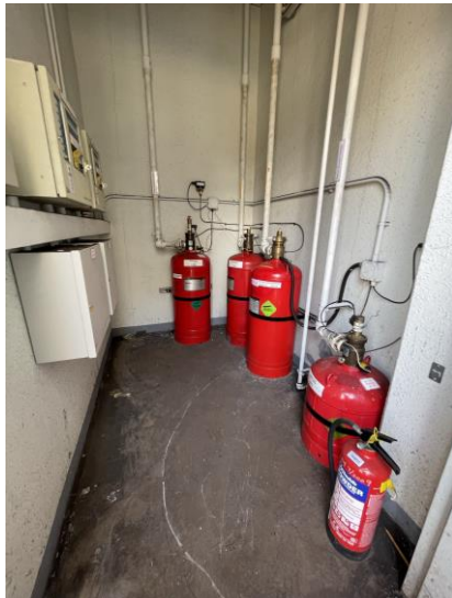
Photo 76: FM-200 cylinder room in Unit 2 FGD Electrical and Control Equipment Building 照片 76 : 二號煙氣脫硫裝置電氣及控制設備機樓的FM-200瓶儲存室
