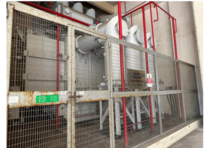
Photo 54: Transformer along the Main Station Building 照片 54 : 沿L1至L3號機組的主廠房大樓的變壓器
