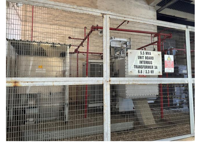
Photo 57: Transformer along the Main Station Building 照片 57 : 沿L1至L3號機組的主廠房大樓的變壓器
