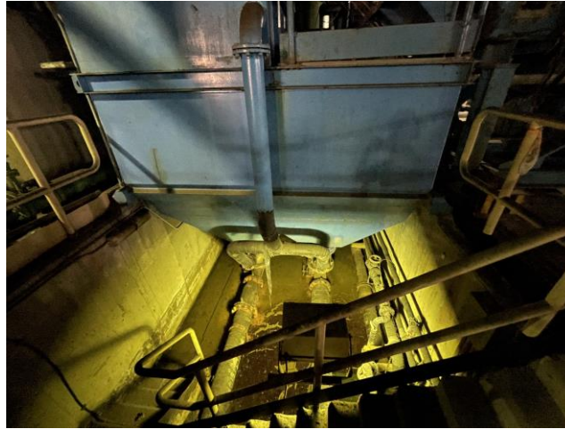
Photo 8: A furnace bottom ash storage bin pit 照片8：爐底灰貯存桶坑
