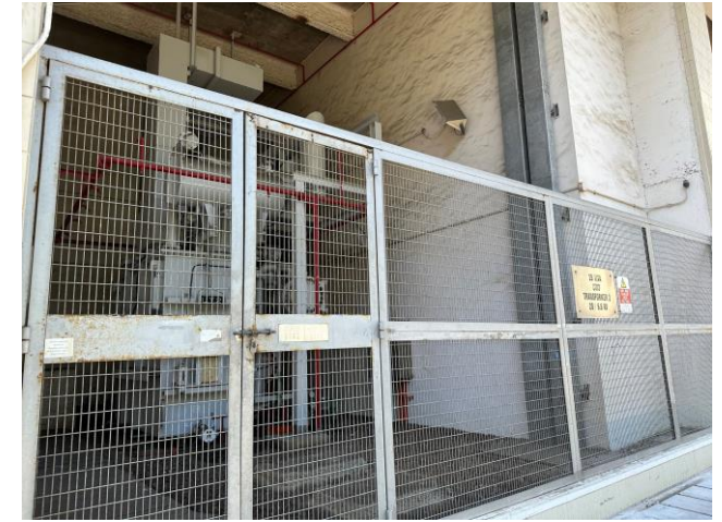
Photo 51: Transformer along the Main Station Building 照片 51 : 沿L1至L3號機組的主廠房大樓的變壓器
