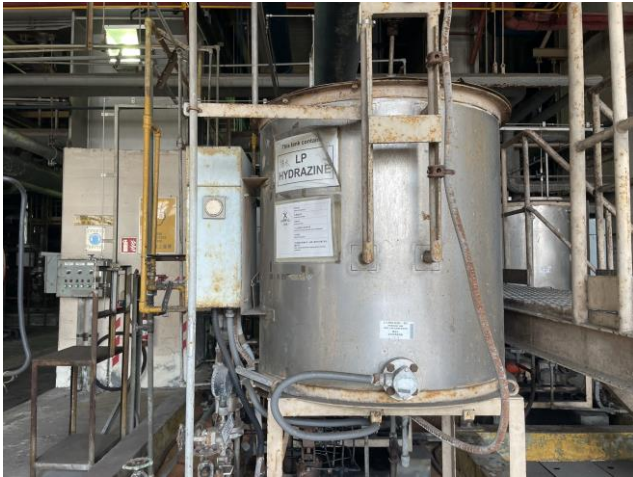
Photo 19: A Hydrazine tank at the chemical dosing system 照片 19 : 化學劑投配系統的聯胺缸
