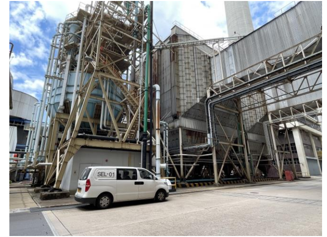
Photo 63: Electrostatic precipitator systems connecting from the Main Station Building for L1 to L3 照片 63：連接L1至L3號機組的主廠房大樓的靜電除塵系統
