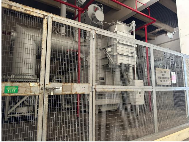
Photo 55: Transformer along the Main Station Building 照片 55 : 沿L1至L3號機組的主廠房大樓的變壓器
