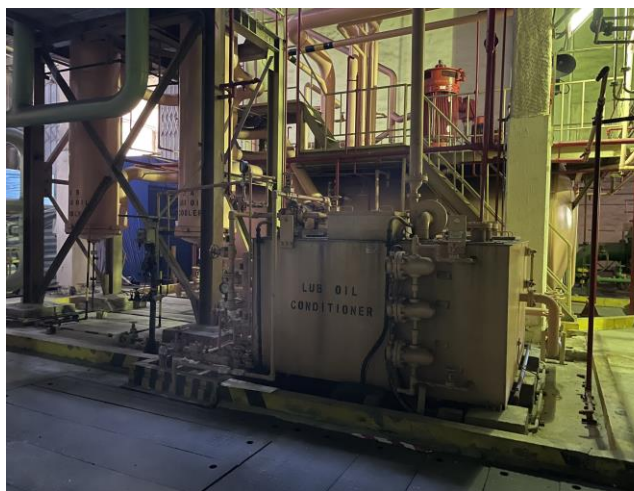
Photo 29: Lubrication oil conditioner and coolers at L2 照片 29 : L2號機組的潤滑油調節器及冷卻器
