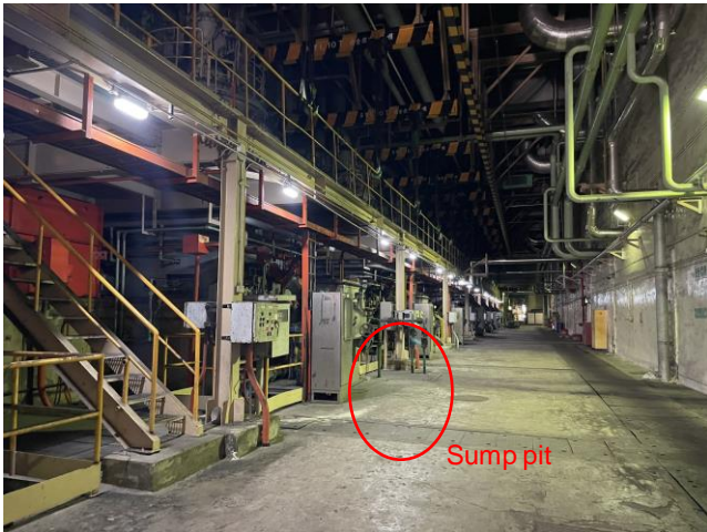
Photo 16: A series of coal grinding mills along the Main Station Building for L1 to L3 and sump pit 照片 16 : 沿著L1至L3號機組的主廠房大樓及集水坑的一列碾煤機
