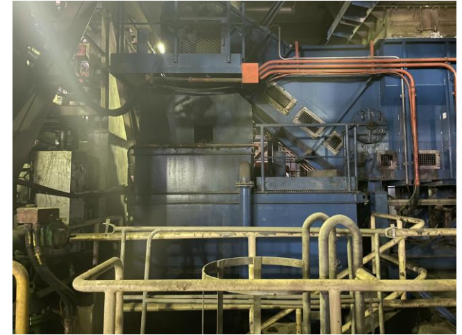
Photo 9: Boiler area and submerged scraper conveyor 照片9：鍋爐區及水下刮板輸送帶
