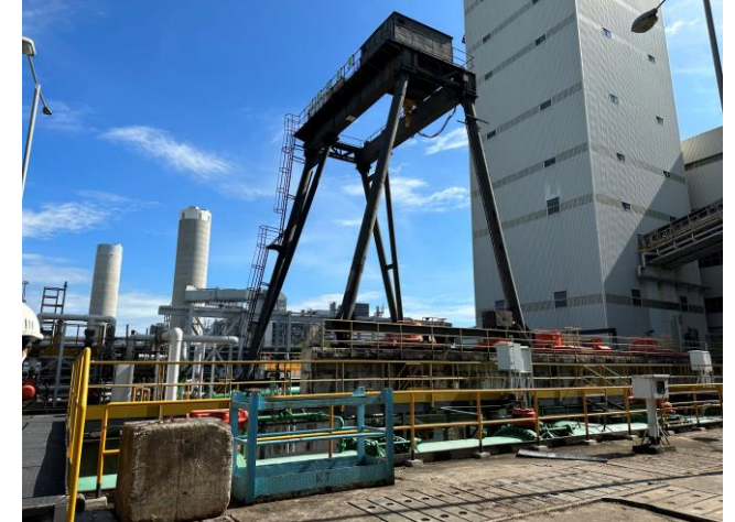
Photo 84: Overview of the circulating water system and Junction Tower T16 at the back 照片 84：循環水系統的概觀和後面的T16號接駁塔
