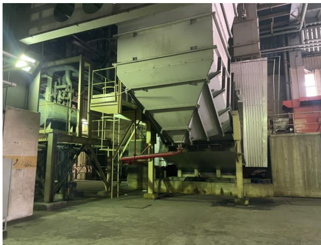
Photo 38: A oil stain near a forced draft fan unit in L2 照片 38：L2號機組內一個鼓風機附近的油漬
