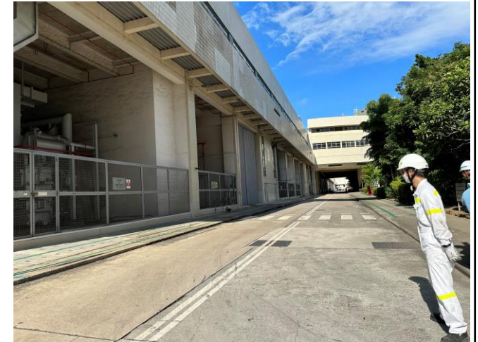
Photo 60: Transformer units along the Main Station Building 照片 60 : 沿L1至L3號機組的主廠房大樓的變壓器組
