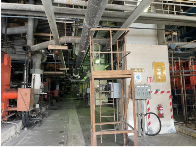
Photo 43: Area near the boiler feed pumps 照片 43：鍋爐給水泵附近區域
