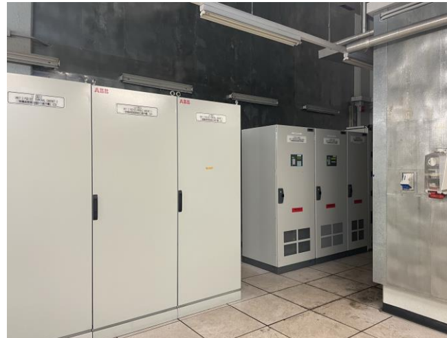
Photo 77: Control equipment room in Unit 2 FGD Electrical and Control Equipment Building 照片 77 : 二號煙氣脫硫裝置電氣及控制設備機樓的控制設備室
