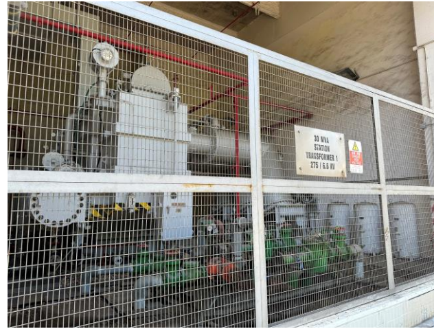
Photo 50: Transformer along the Main Station Building 照片 50 : 沿L1至L3號機組的主廠房大樓的變壓器
