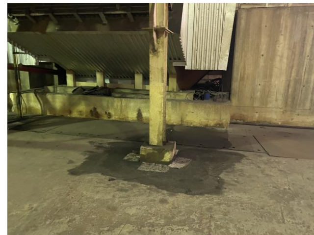
Photo 39: A oil stain near a forced draft fan unit in L2 照片 39：L2號機組內一個鼓風機附近的油漬
