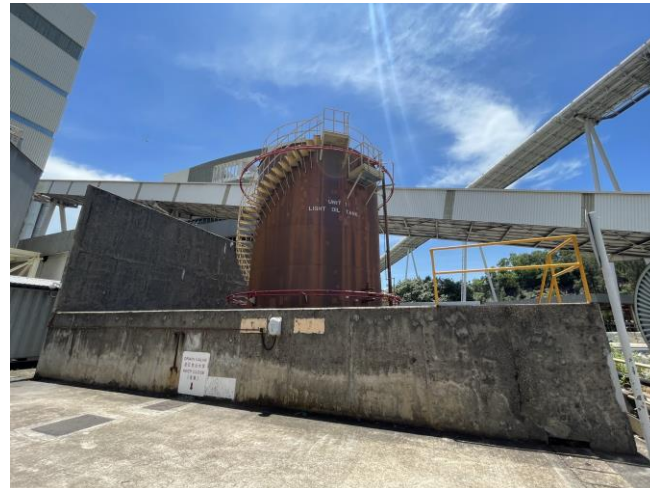
Photo 71: Secondary containment of Unit 1 Light Oil Tank 照片 71：一號輕質油儲存缸的次層密封區
