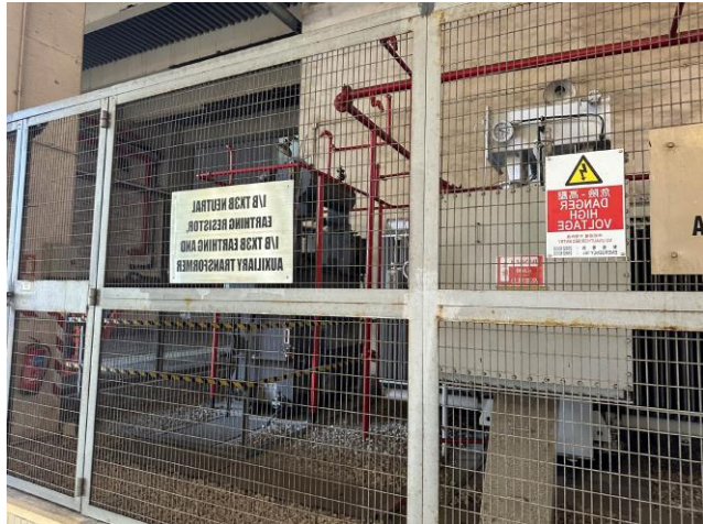
Photo 58: Transformer along the Main Station Building 照片 58 : 沿L1至L3號機組的主廠房大樓的變壓器
