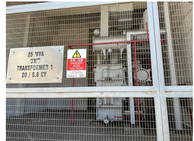
Photo 48: Transformer along the Main Station Building for L1 to L3 照片 48：沿L1至L3號機組的主廠房大樓的變壓器
