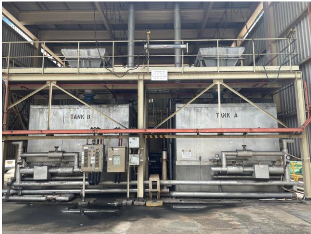
Photo 82: Two Sulphur melting / store tanks underneath a shelter with oil stain observed 照片 82：兩個簡棚下的溶硫／儲硫缸（觀察到有油污）
