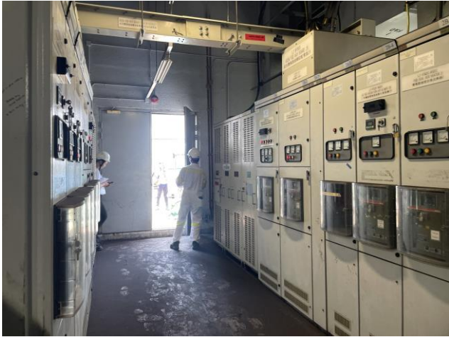
Photo 79: Switchgear room in Unit 2 FGD Electrical and Control Equipment Building 照片 79：二號煙氣脫硫裝置電氣及控制設備機樓的開關設備室
