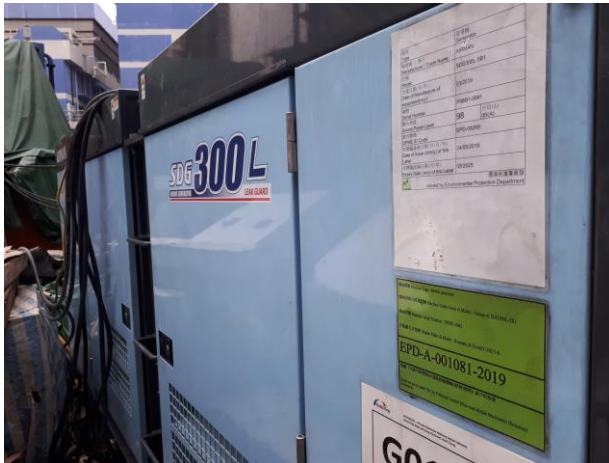
Figure A2 NRMM label on Generator
