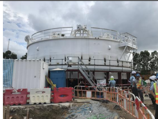
Bio Gas Tank
