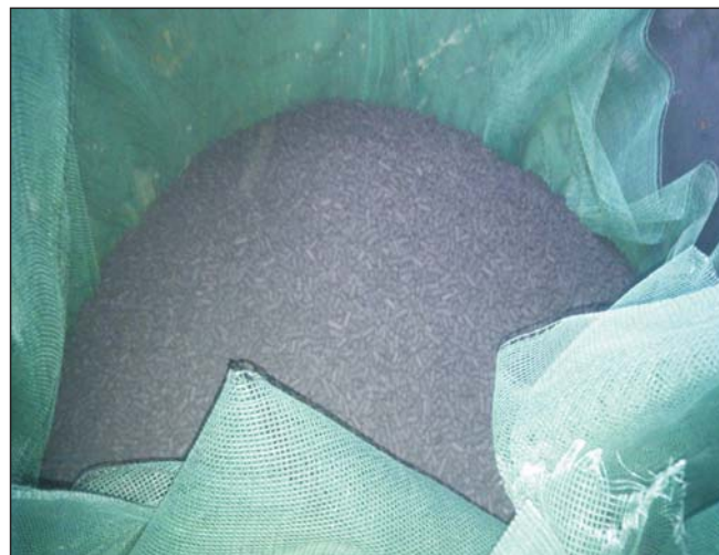
Photo 14: Activated charcoal placed at the exhaust drum of the blower
