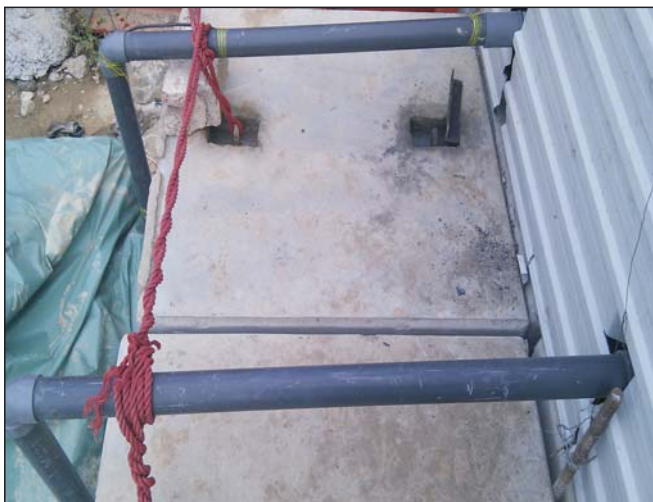
Photo 13: Aeration piping connecting the biopile to the blower
