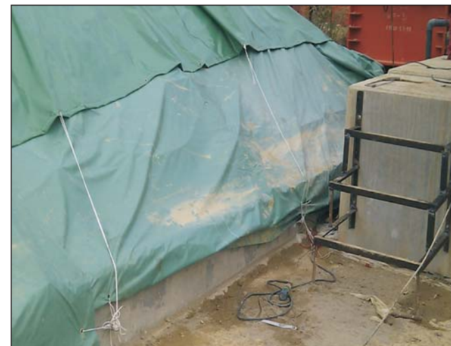
Photo 12: Tarpaulin sheeting affixed to the metal hook
