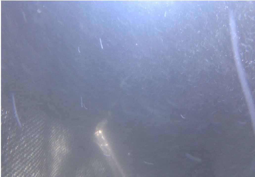
Fig. 10 Geotextile Condition of Silt Curtains
