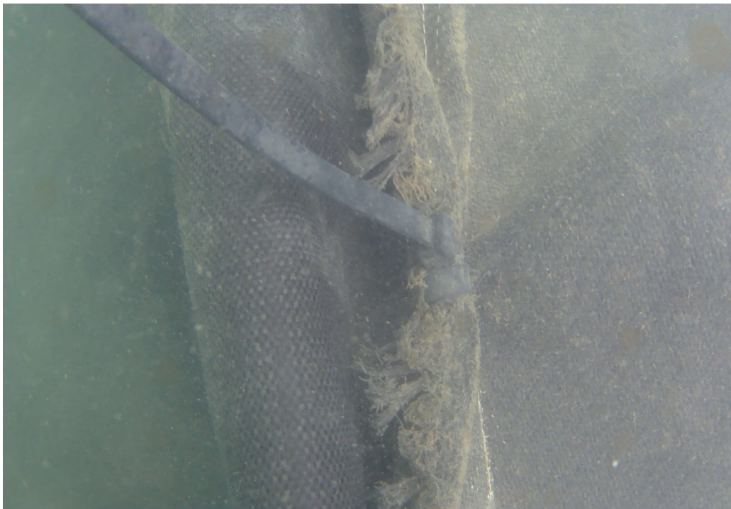
Fig. 11 Geotextile Condition of Silt Curtains
