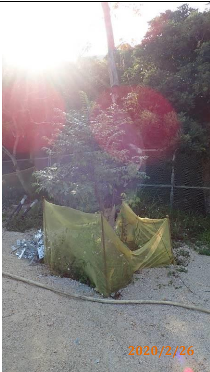
Photo 11. Collapsed fence shall be promptly rectified.
