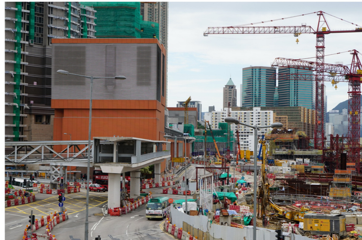
VC19 (LCA10) Guangzhou-Shenzhen-Hong Kong Express Rail Link (XRL) Terminus Construction Site and Austin Station
