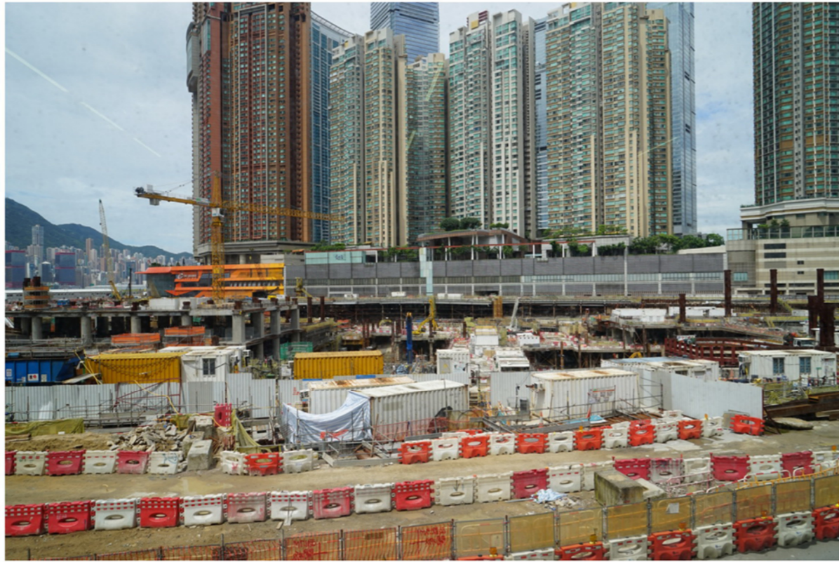
VC20 (LCA10) Guangzhou-Shenzhen-Hong Kong Express Rail Link (XRL) Terminus Construction Site and Austin Station 5-8-2014
