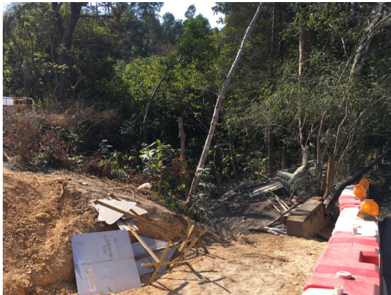
Description: Contractor was reminded to extend the protective fencing for Keteleeria fortunei .
