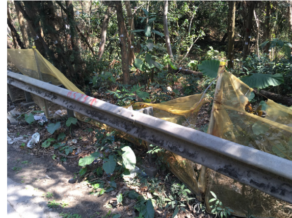
Description: Contractor was reminded to keep maintain the protective fencing properly and replace the loosing fencing for Keteleeria fortunei .
