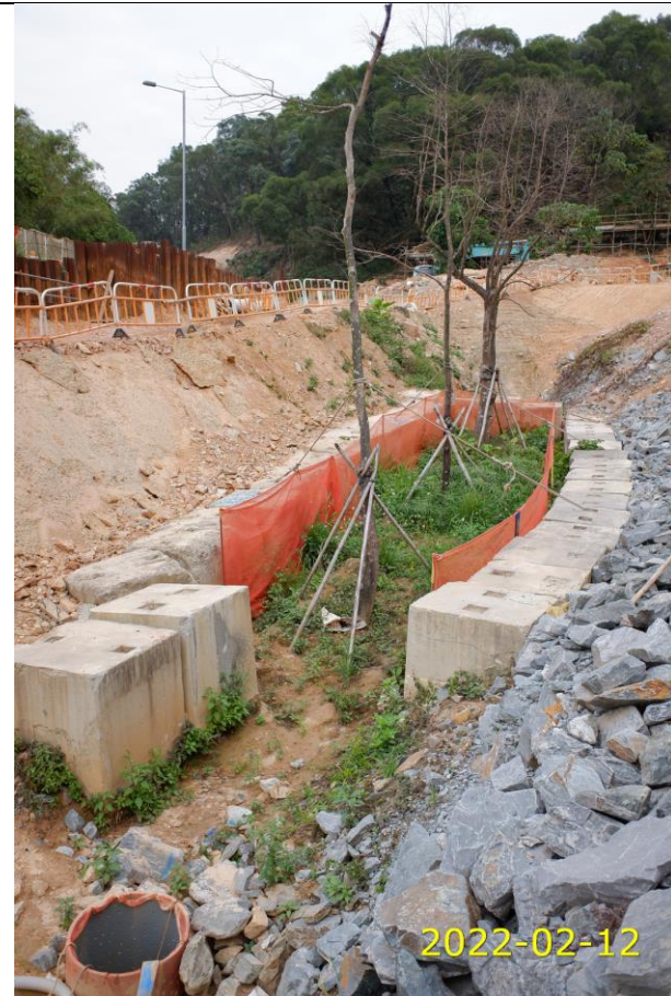
Formation of ditch to guide surface runoff to water pumping location, moist soil surface observed
