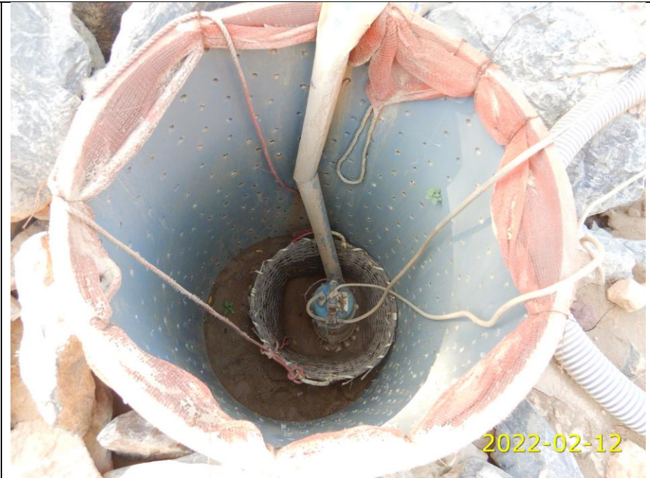
Submersible pump standby
