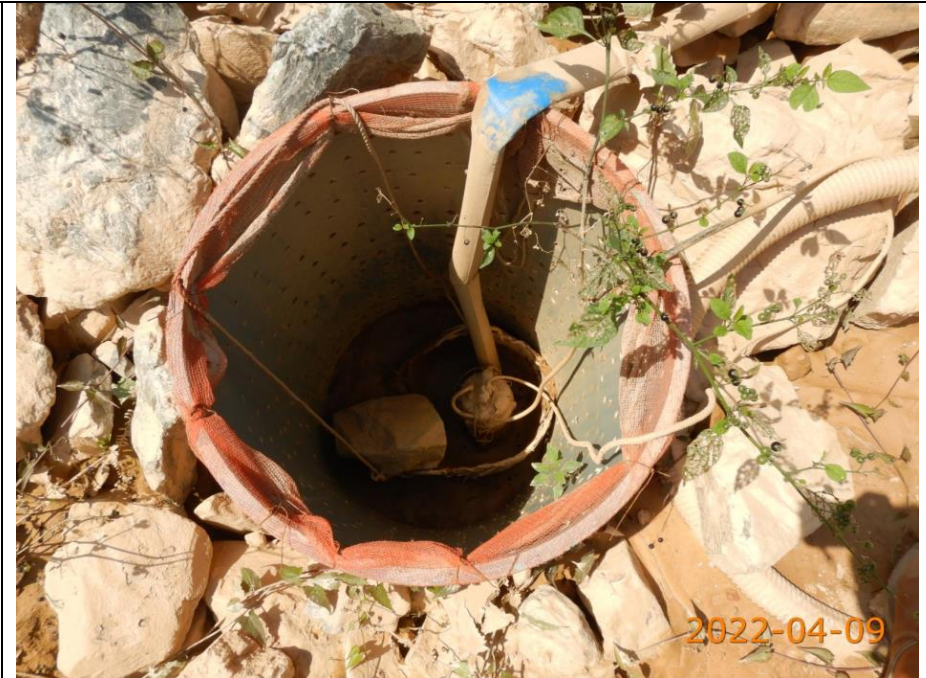
Submersible pump standby
