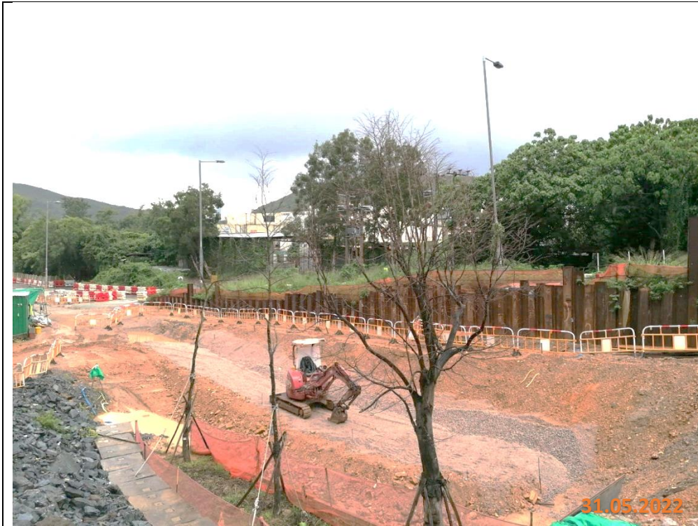
Formation of ditch to divert the surface runoff into water collection point
