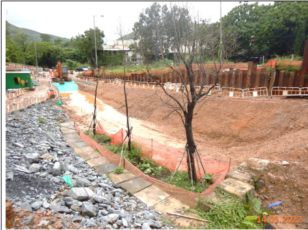
Formation of ditch to divert the surface runoff into water collection point
