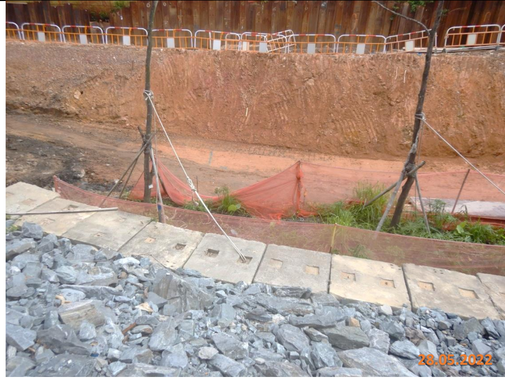
Formation of ditch to divert the surface runoff into water collection point
