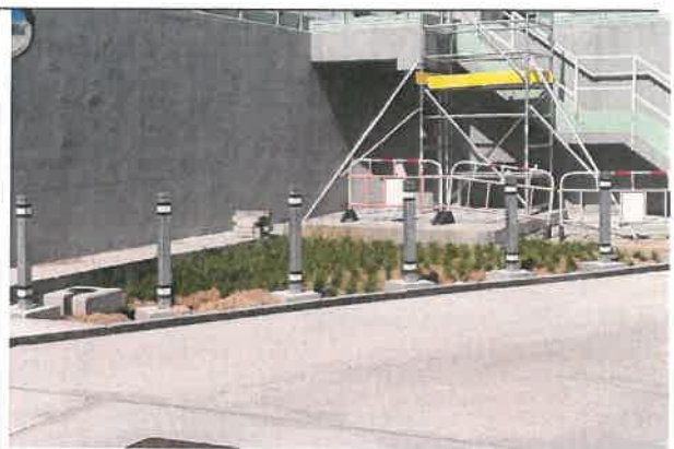
Planting works affected by other works still require reinstatement
