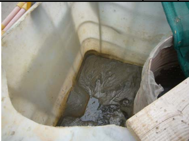
Photo 3: Poor performance of de-silting tank was observed at Tai Shiu Ha works area, the contractor was reminded to improve the de-silting facility.
