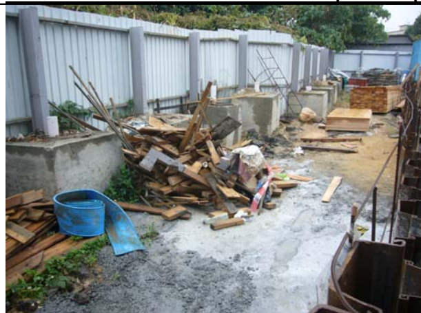
Photo 2: C&D waste cumulated on site was observed at Shui Tsui San Tsuen Pumping Station, the contractor was reminded to dispose the waste in regular basis.
