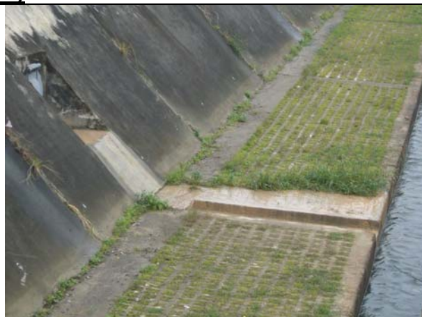
Photo 3: Turbidity water discharged from the Tai Shiu Ha works area was observed, the contractor was requested to improve the de-silting facility immediately to prevent discharge of turbid water.
