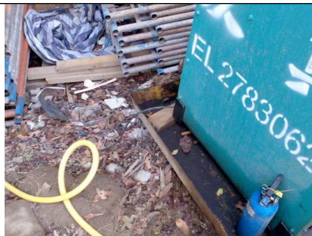
Stagnant water inside the drip tray was cleared.
