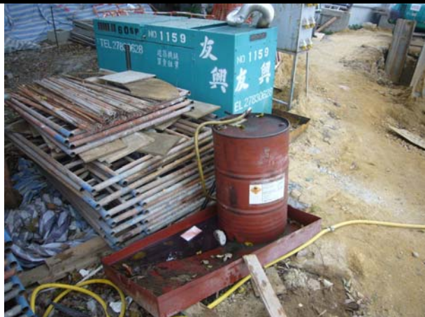
Photo 1: Stagnant water was observed within the drip tray. The Contractor was reminded to clear water to prevent mosquito breeding. (STSTPS)
