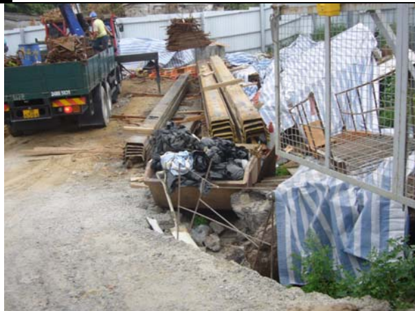
Photo 2: General and C&D waste cumulated was observed, the contractor was reminded to clean in regular basis. (STSTPS)
