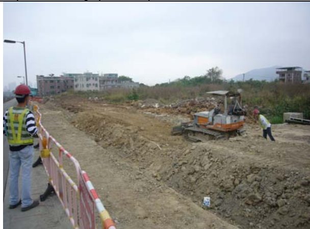
Photo 3: Stockpile at Kiu Hing Road without cover was observed, the contractor was reminded to provide proper mitigation measures to prevent dust generation.
