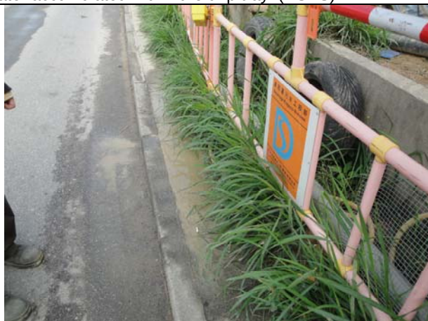
Photo 3: Some slurry was observed along the site boundary. The contractor was reminded to maintain good practice to confine and treat the waste water in order to prevent direct discharge of waste water.
