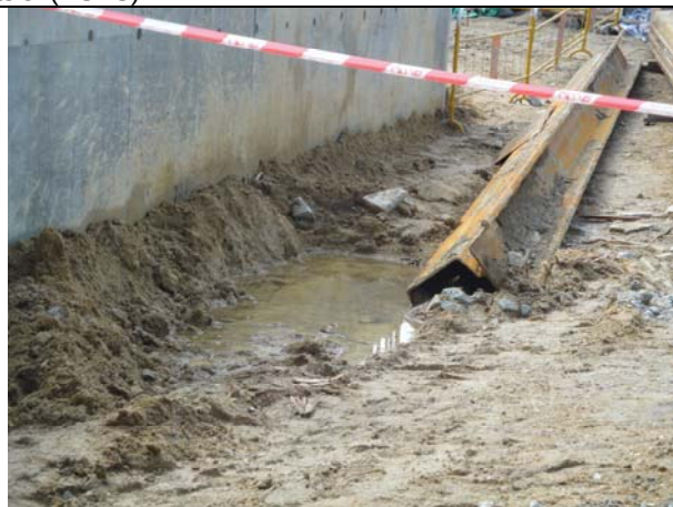
Photo 4: Some stagnant water was observed. The contractor was reminded to implement proper measures to alleviate the potential impact of mosquitoes breeding. (STSTPS)
