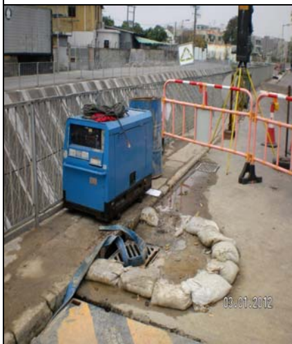
Photo 3 Generators without drip trays
