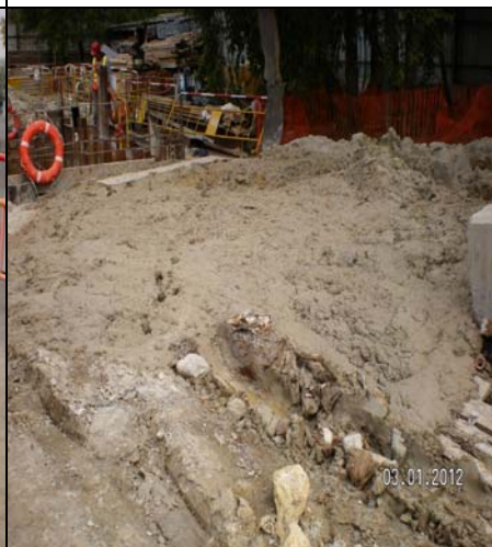
Photo 4 Mud stock piled within the site at Ha Tsuen Pumping Station
