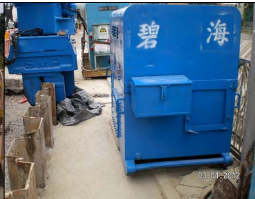
Photo 2 Generators without drip trays
