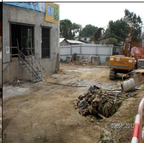
Photo 5 Construction waste stock piled within the site at Shui Tsiu Tsuen Pumping Station.
