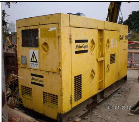
Photo 1 Generators without drip trays
