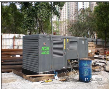
Photo 1: Oil drum without drip tray at Ha Tsuen Pumping Station.
