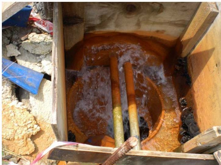
Photo 1: Excessive discharge at Ha Tsuen Pumping Station
