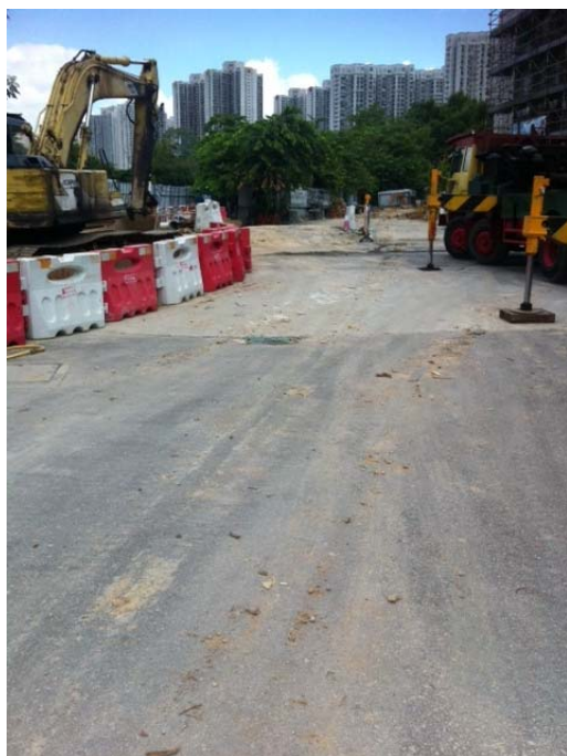
Photo 2: Mud trail was observed at the exit/ entrance of the site of Ha Tsuen Sewage Pumping Station, wheel washing facility should be properly maintained. Also, watering at the site exit should be applied more frequently.
