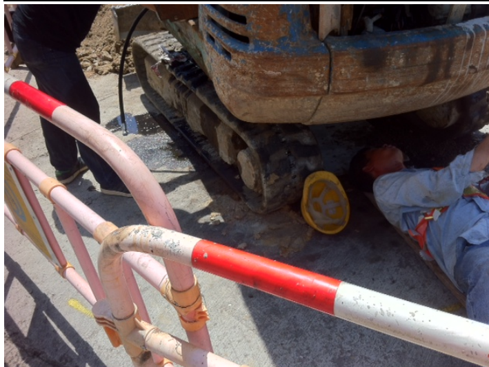
Photo 1: Oil leaking from an idled plant was observed in Tai Shue Ha East Road, the Contractor should clean the oil stain promptly after the maintenance work to avoid potential land contamination.
