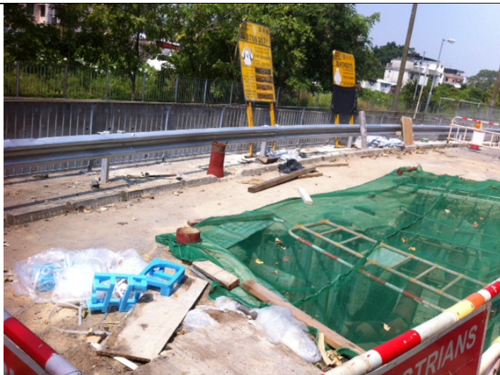
Photo 1: Scattered of C&D waste was observed in Shui Tsui San Tsuen road, the Contractor should improve the housekeeping of the construction site.
