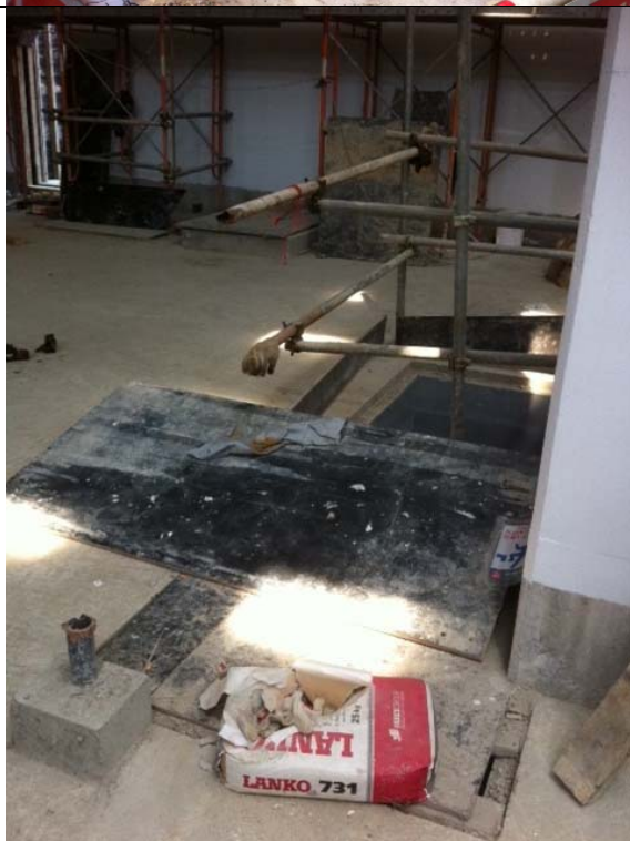
Photo 2: An opened cement bag was observed in Ha Tsuen Sewage Pumping Station, the Contractor should cover it with tarpaulin sheet or other means to prevent fugitive dust or remove it immediately.
