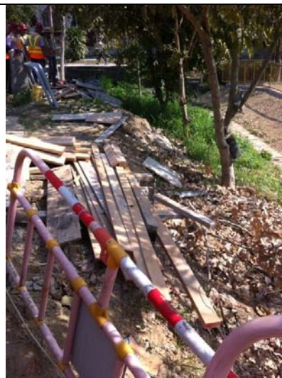
Photo 2: The retained trees in Shui Tsui San Tsuen Road were not fenced off properly, the Contractor should provide proper fencing for it and keep it away from work.
