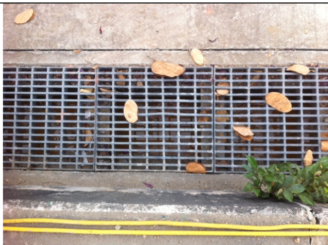
Photo 1: Muddy water and debris in exiting u-channel was observed in Tai Shu Ha Road, the Contractor should clean the u-channel properly to avoid drainage blocking.
