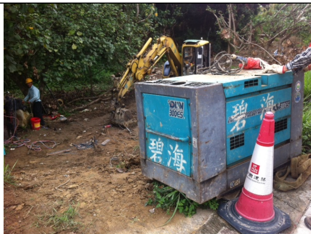
Photo 2: Generator without drip tray was observed in the working area of Shum Chung, the Contractor should provide drip tray underneath.
