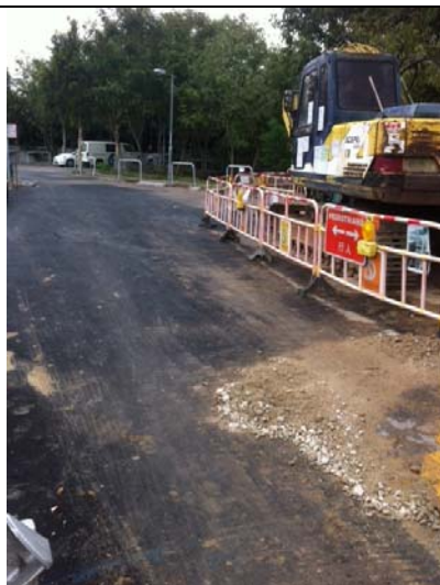
Photo 1: Mud tails was observed in Shui Tsui Sewage Pumping Station, the Contractor should clean it properly.
