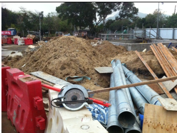
Photo 3: Dusty stockpile was observed in Ha Tsuen Sewage Pumping Station, the Contractor should cover it with impervious sheet or remove it off site properly.
