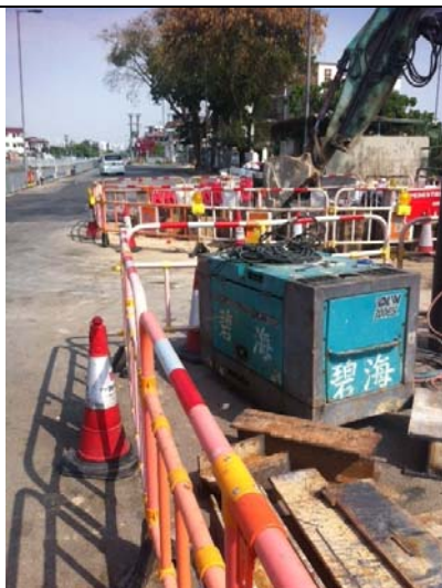
Photo 1: Generator without drip tray was observed in the working area of Hiu Hing Road, the Contractor should provide drip tray underneath.
