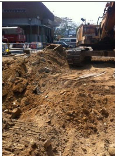
Photo 2: Dusty stockpile was observed in Ha Tsuen Sewage Pumping Station, the Contractor should cover it with impervious sheet or remove it off site properly.
