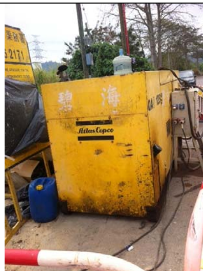
Photo 2: Generator without drip tray was observed in the working area of Hiu Hing Road, the Contractor should provide drip tray underneath.
