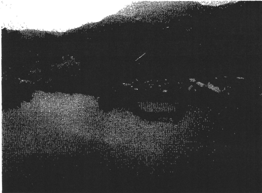
Geotextile linings along the bank of Ho Chung River were found removed in our inspection on 14.03.08.
