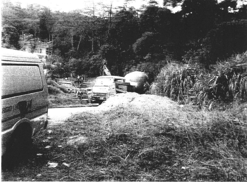
Photo 3: Concreting works was undergoing at another construction site in the upstream area.
