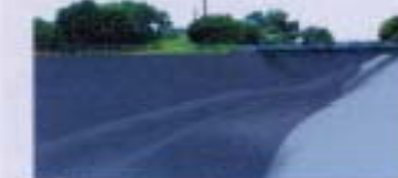
Drainage channel with concrete lining only -unsightly
