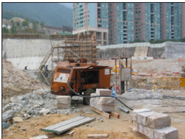
Figure 6-2 – The air compressor near Monte Vista.
