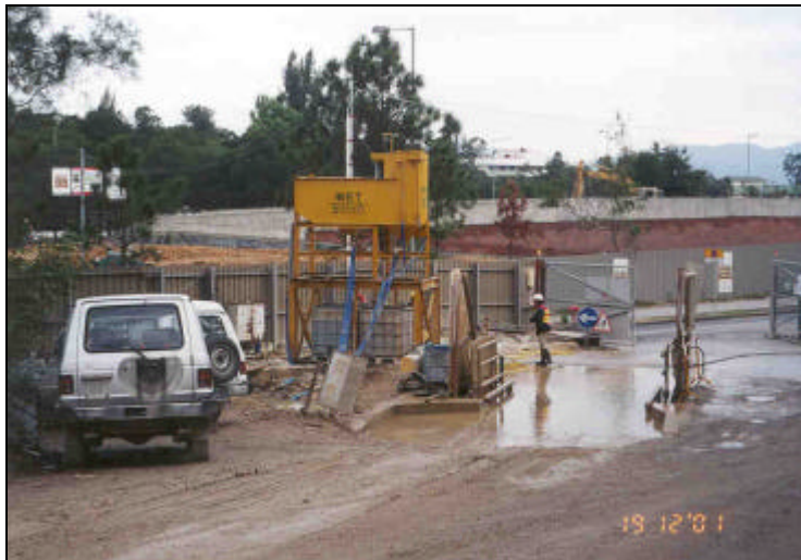
Figure 6-1 The wastewater treatment facility at site entrance near Cheung Muk Tau Village.
