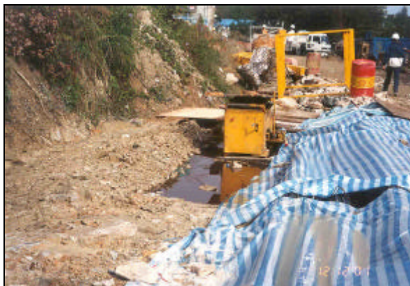
Figure 6-2 The oil spillage at Portal D area.
