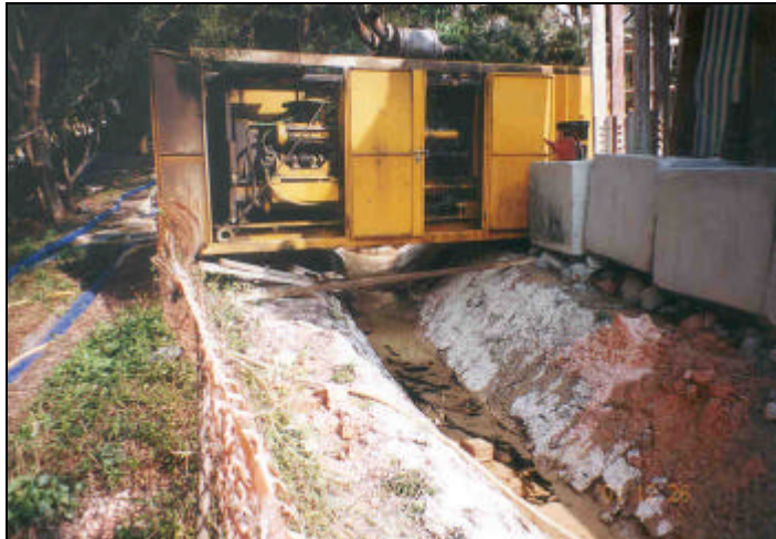
Figure 6-4 The pollutants generated from a generator.
