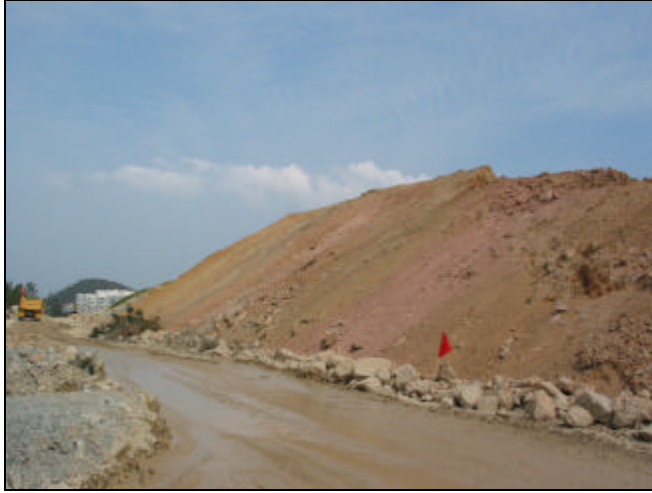
Figure 6-3 – The exposed slope of stockpile near Monte Vista.
