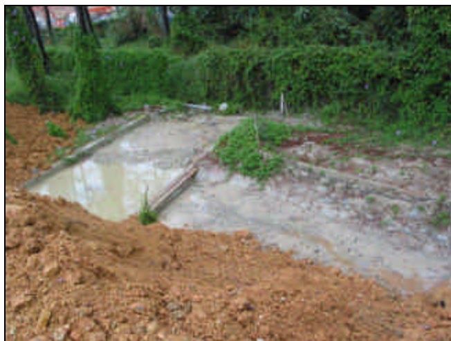
Figure 6-2 – The excavated material and silty water at the channel near Portal D area.
