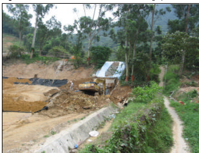
Figure 6-2 – The blocked inlet channel of discharge point No. 6.
