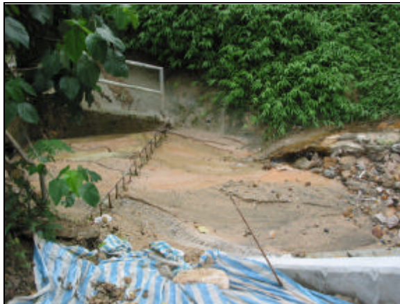
Figure 6-1 – The silty channel near stream S28.
