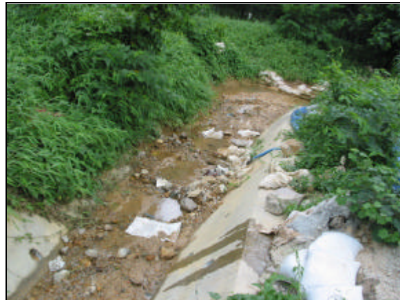
Figure 6-2 - The silty channel at discharge point no. 6
