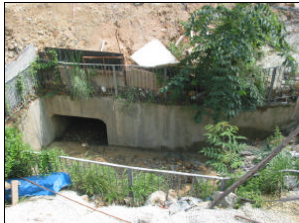
Figure 6-2 - The silty channel at discharge point no. 7
