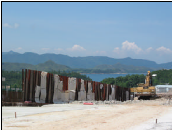
Figure 6-5 - The broken portable noise barriers near Monte Vista.
