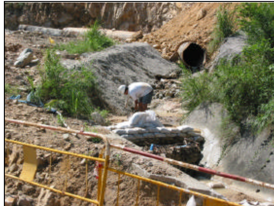
Figure 6-2 - The cleaning work in progress for silty channel along discharge point no. 7
