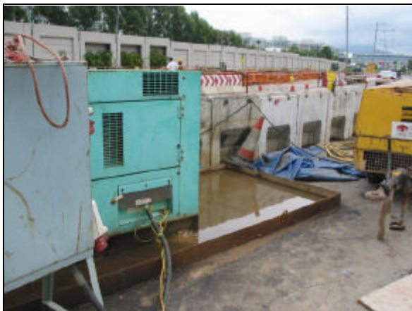
Figure 6-3 – Stagnate water in drip tray.
