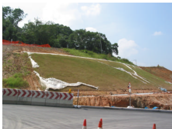
Figure 6-4 - The exposed slope near discharge point no.3
