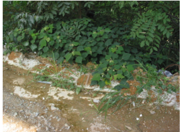
Figure 6-6 - Sandbags for flood protection were damaged.
