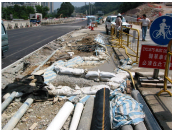
Figure 6-7 - Sand trap of the wheel washing bay in casting yard.
