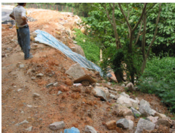
Figure 6-3 - The exposed slope near discharge point no. 6
