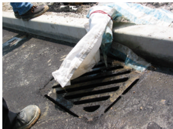
Figure 6-8 - Slit was discharged into road gully.
