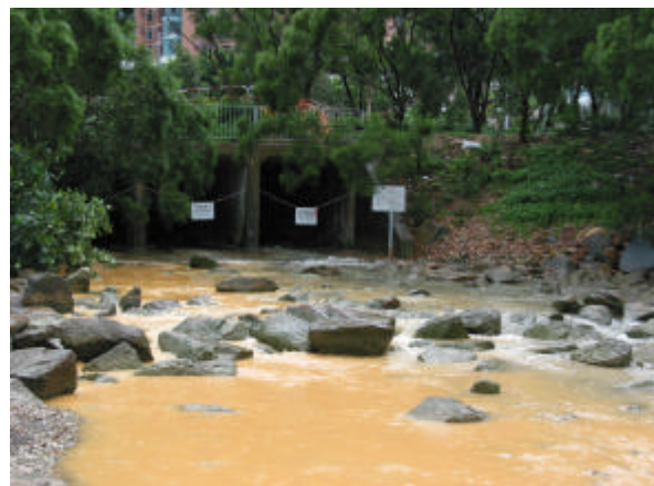
Figure 6-2 - Muddy runoff flow through box culvert besides Wu Kai Sha Youth Village
