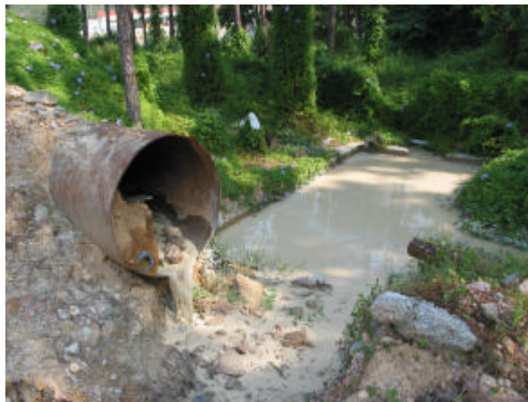
Figure 6-1 - Surface runoff near discharge point no. 8
