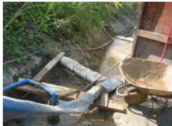
Figure 6-4 - Sand trap is now well maintained.
