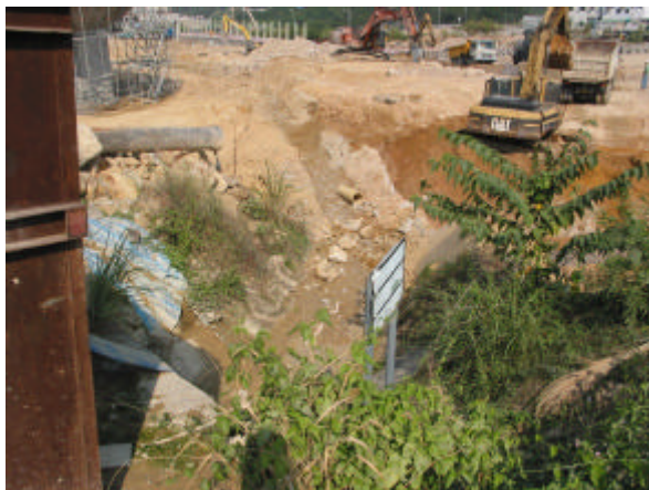
Figure 6-3 - Drainage channel S3 was not well maintained.
