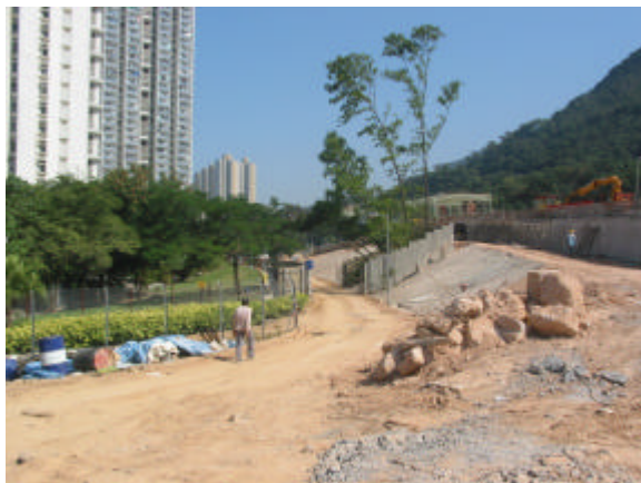
Figure 6-5 - Unpaved road at Area J21B.
