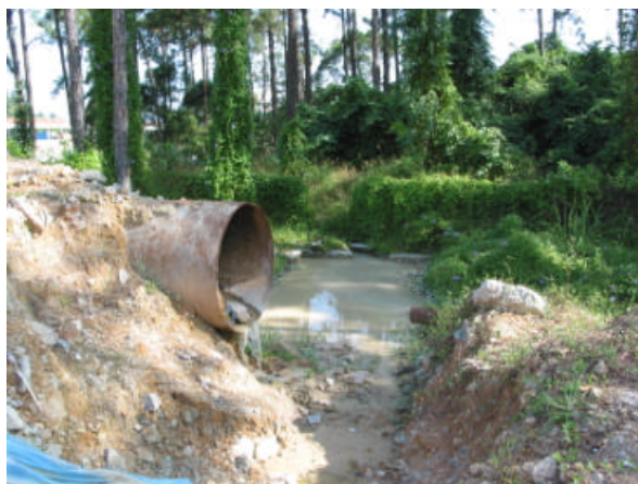
Figure 6-1 - Surface runoff near discharge point no. 8
