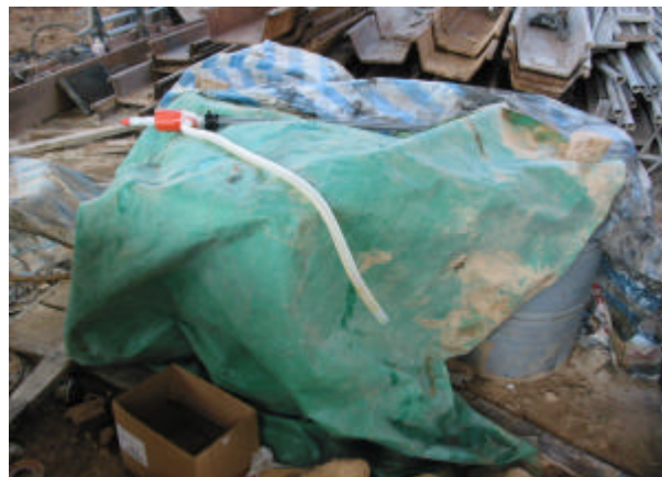
Figure 6-6 - Oil drums was not provided with drip trays.
