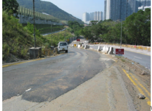
Figure 6-4 - Muddy water on Leung Yau Road.
