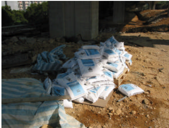
Figure 6-3 - Cement bags uncovered.
