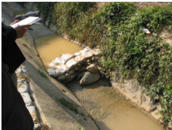
Figure 6-1 - Silty channel at Discharge Point 6.
