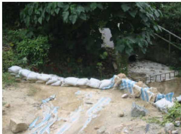
Figure 6-2 - Damaged sandbags near channel S28 & S29
