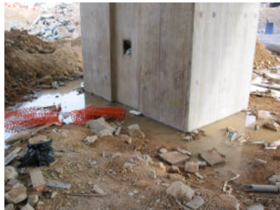
Figure 6-6 - Stagnant water under Bridge D.
