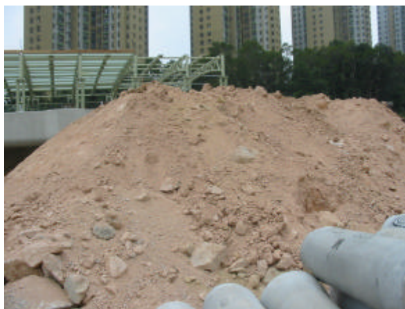
Figure 6-2 - Exposed slope near Discharge Point 3.
