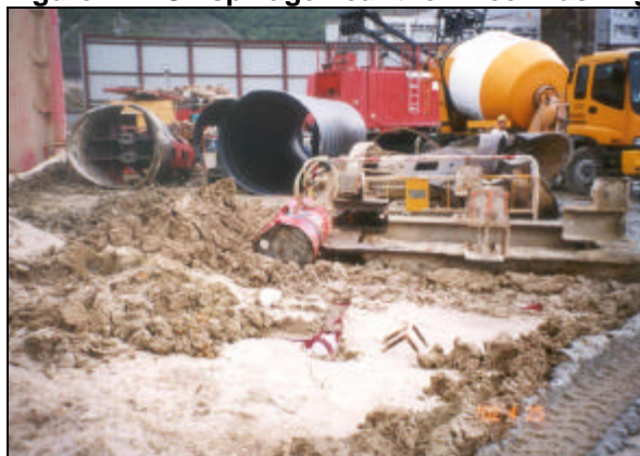
Figure 2 Oil spillage near the wheel washing bay
