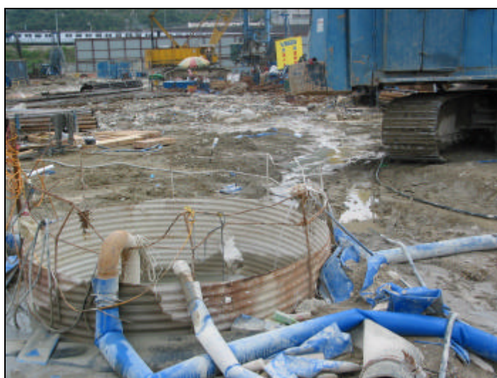
Figure 6-1 Site runoff was collected in the pre-treatment tank.
