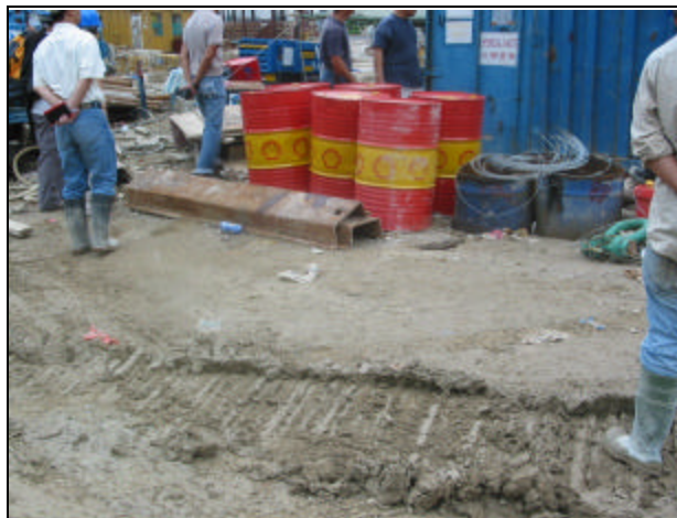
Figure 6-1 Diesel drums placed at open area.
